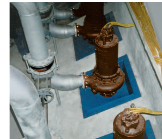
Sewage pumps installed dry.
