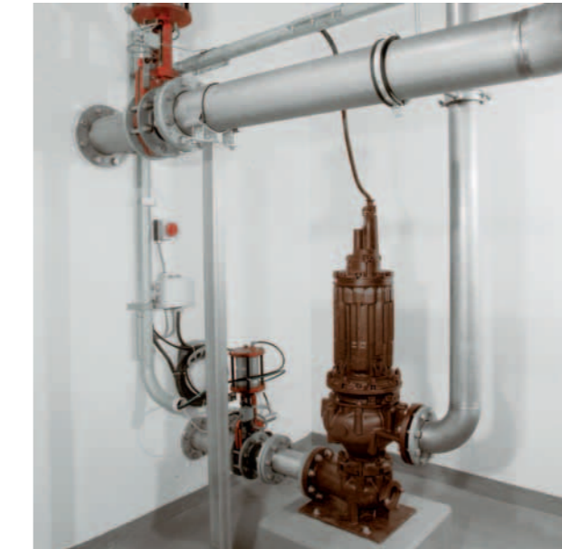
Sludge pumps with a special suction stand installed vertically and dry.
